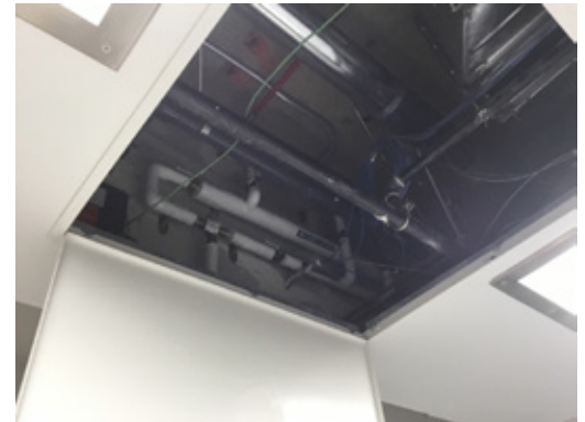
Properly sealing all penetrations is critical to maintain relative room pressures.
